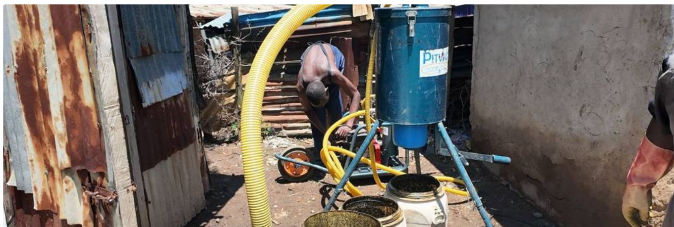
A PitVaq in a dense Kisumu settlement. Narrow access, corrugated iron walls, barrels filled on site. This is the reality vacuum trucks cannot serve.
